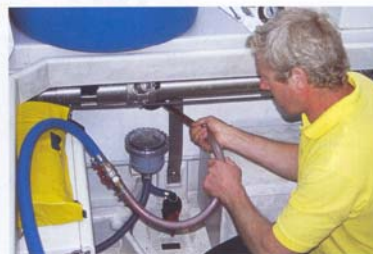
above A rigid, angled pipe is inserted through the access hole to suck fuel up from the bottom of the tank and circulate it.
